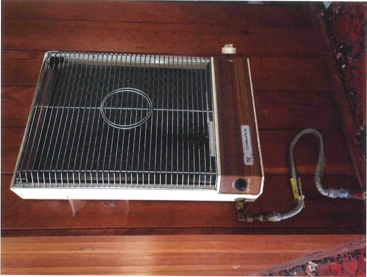
picture, heating system
